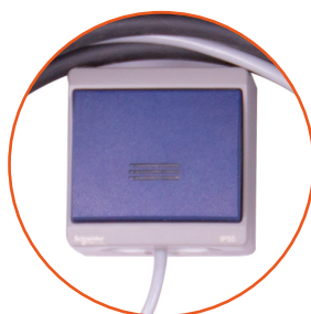
Eclairage gaine piloté par Bus CanOpen Lift Shaft lighting managed by Bus CanOpen lift
